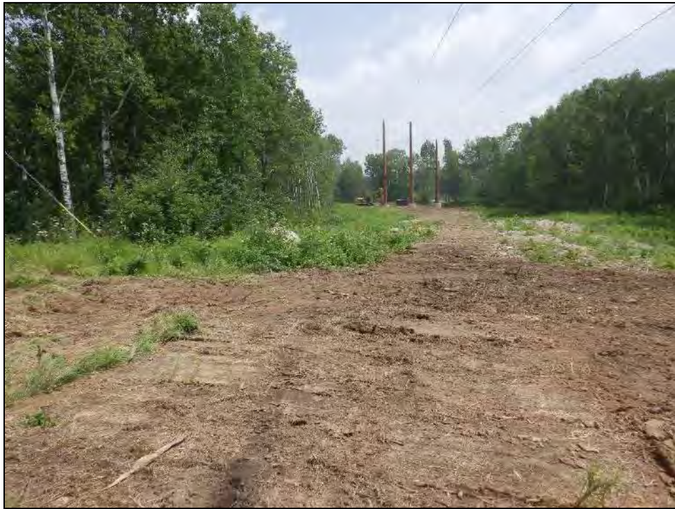
Figure 110E: View of typical disturbed conditions (construction activity) within the project area (R0016567/R0016562).
