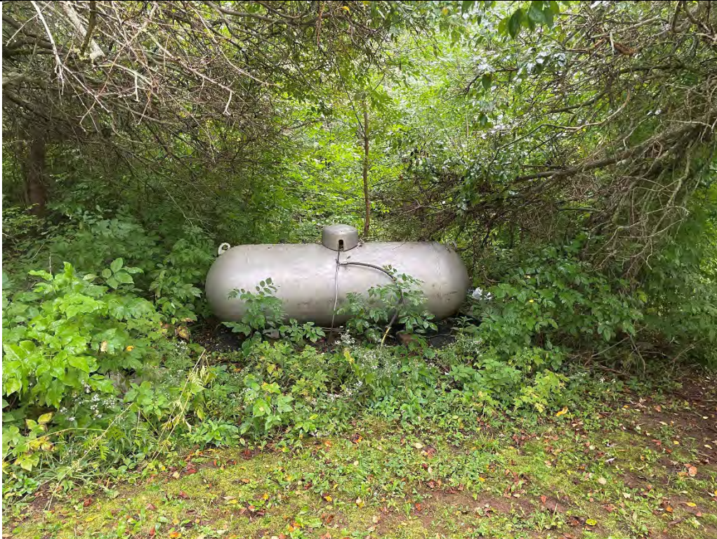
Photograph 3 September 11, 2025 Direction: South Subject: Propane tank (3635)
