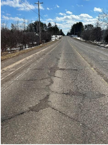
Example of Fatigue cracks
