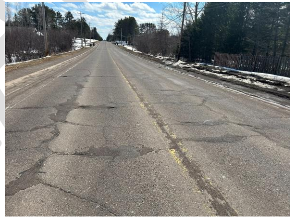
Example of Longitudinal cracks
