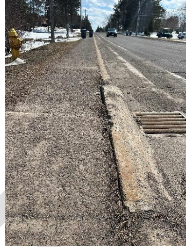
Damaged Curb & Gutter
