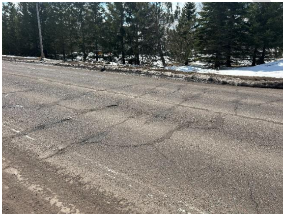
Example of Transverse cracks
