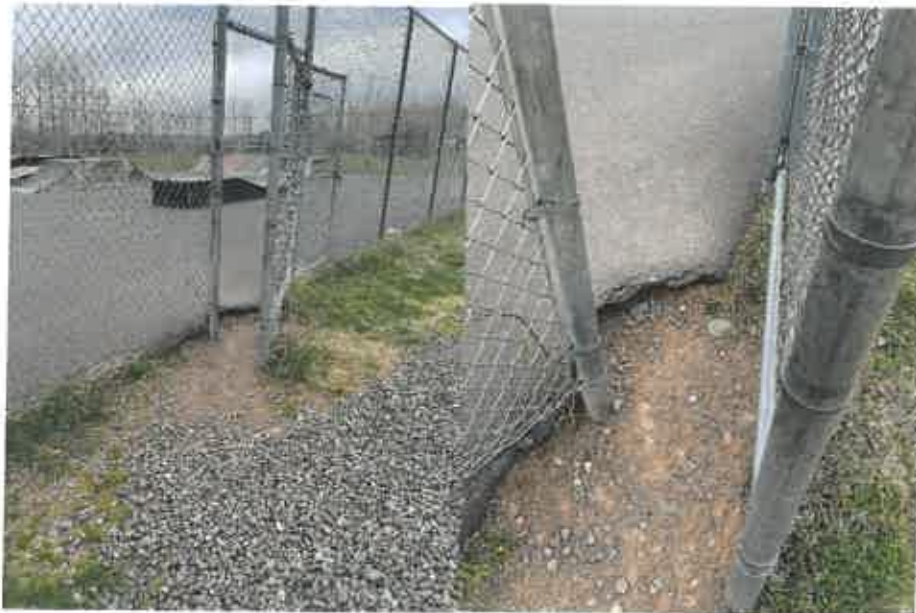
Fence opening is not ADA compliant. Excessive grade change at pavement entry
