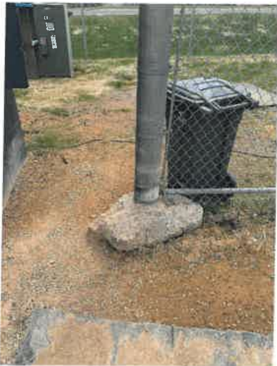
Potential trip hazard – how to address?
