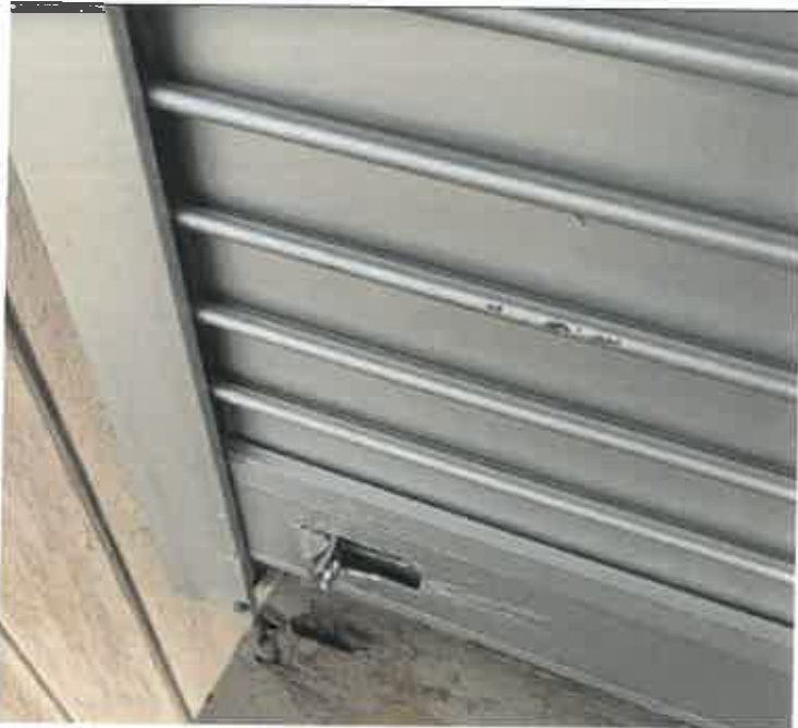
Damage to sliding door mechanism. Work with HYBB to address
