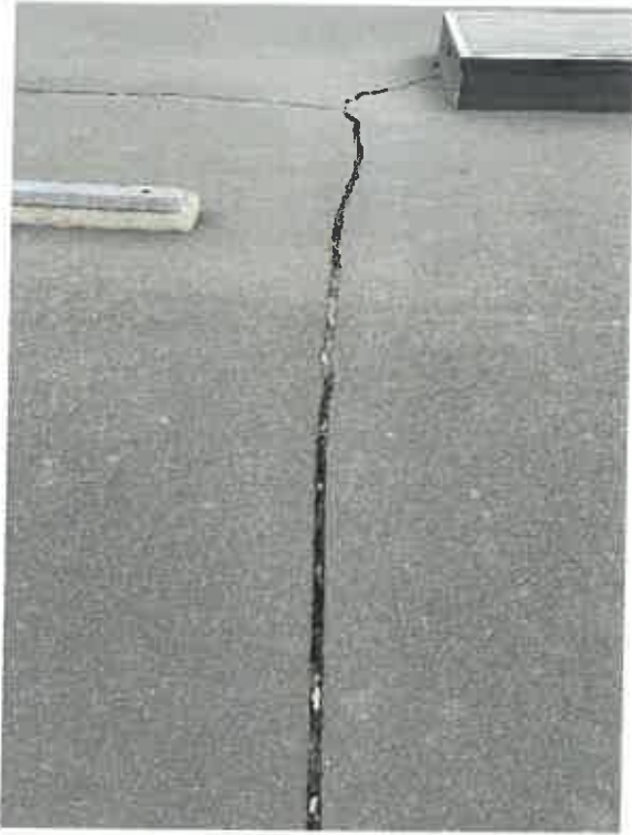
Seal cracks. Budget for eventual replacement
