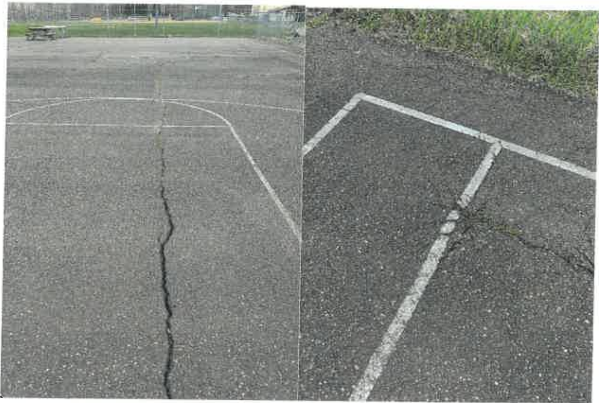
Seal cracks. Budget for eventual replacement
