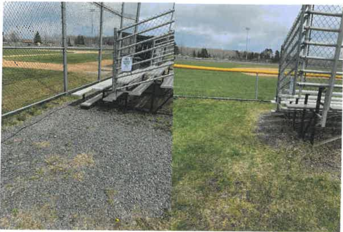
Accessibility to bleachers needs to be considered
